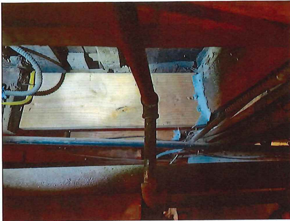
Photo showing additional floor joists to support damage floor joists under underlayment in bathroom on first floor.
