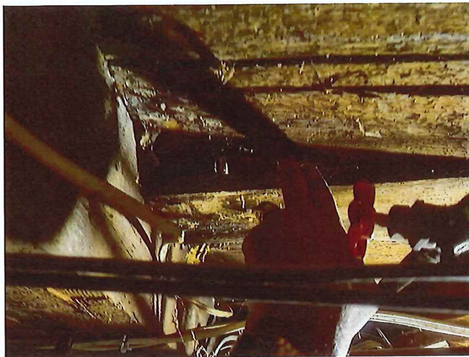
Photo showing deteriorating floor underlayment in bathroom on first floor.
