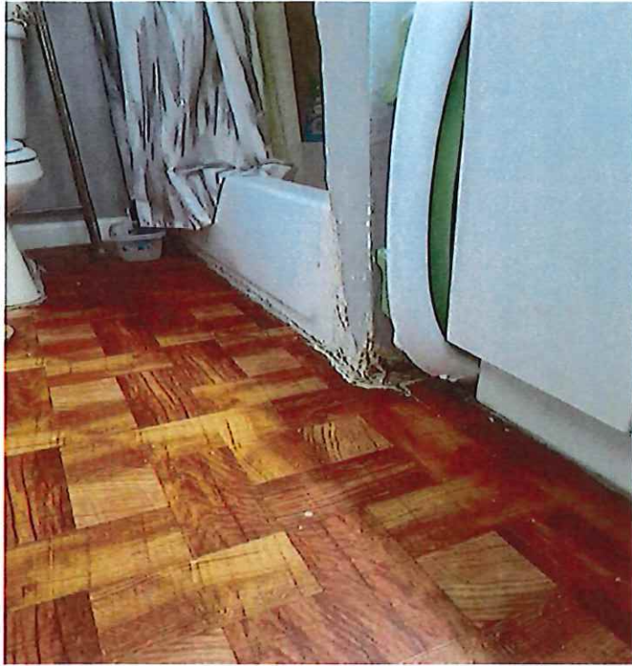
Photo showing deteriorating floor in bathroom on first floor and uneven floor in bathroom on first floor.
