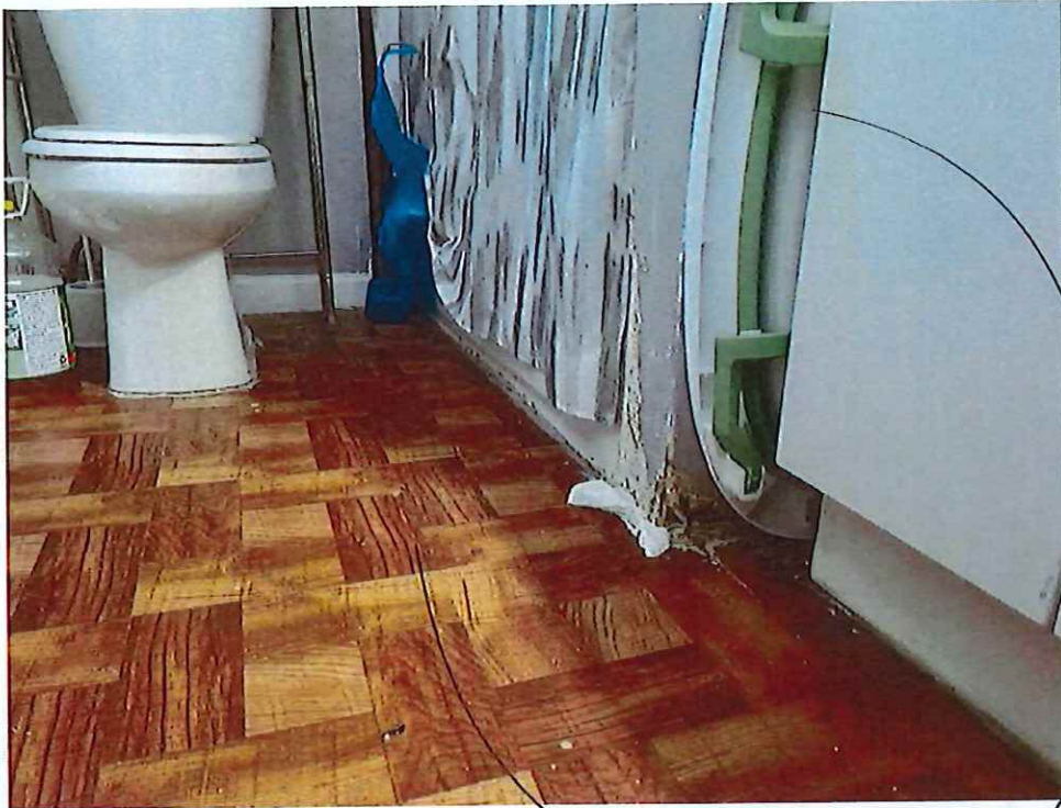
Photo showing deteriorating floor in bathroom on first floor and uneven floor in bathroom on first floor.
