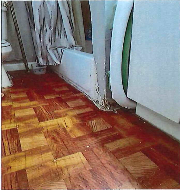
Photo showing deteriorating floor in bathroom on first floor and uneven floor in bathroom on first floor.
